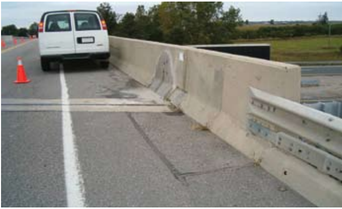
Fig. 1: Cores were taken from the barrier wall of the Chatham Bridge in Chatham, ON, Canada
