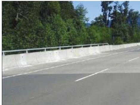
Fig. 2: Cores were taken from the barrier wall of the Waterloo Creek Bridge on Vancouver Island, BC, Canada
